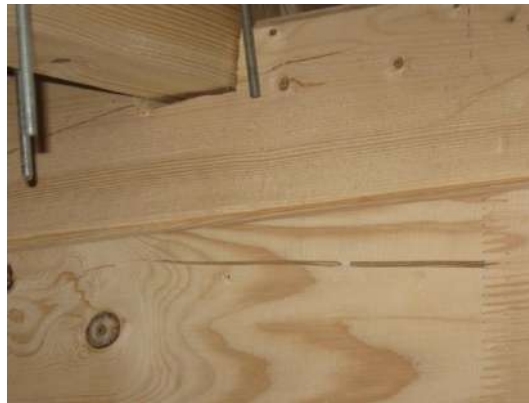
Figure 5.56: Cracks seen near the intersection of the floor beams with the log wall
