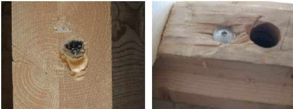
Figure 5.53: Chipping of wood around screws
