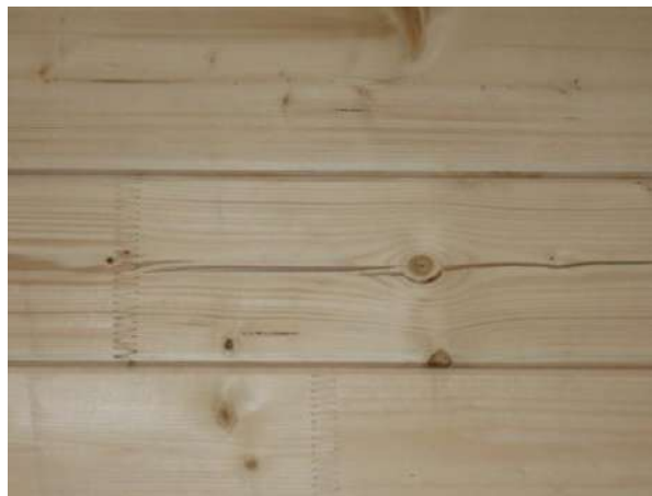
Figure 5.50: Crack seen along the grain of the log
