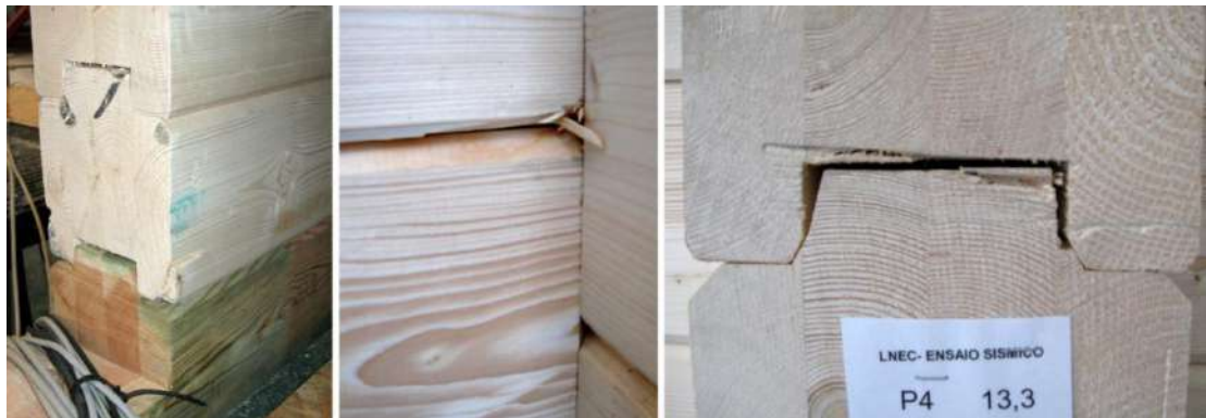
Figure 5.55: Damage to the top and bottom profiles of the log
