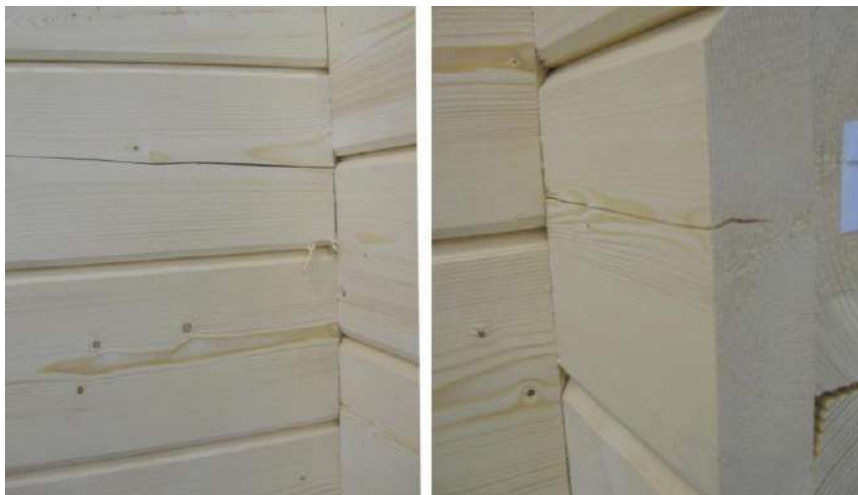
Figure 5.51: Cracks seen in logs at cross wall intersections
