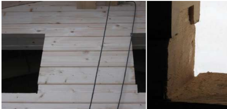
Figure 5.52: Sliding of logs near the window openings in the NW part of the house
