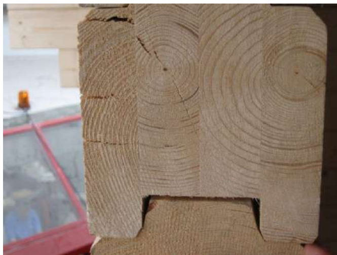
Figure 5.54: Cracks visible in the cross section of the log
